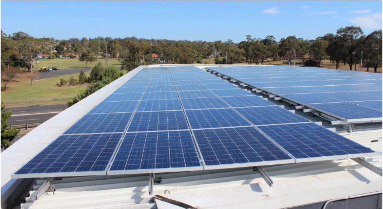
Solar Panels on Campbelltown Arts Centre. Source: Campbelltown City Council
