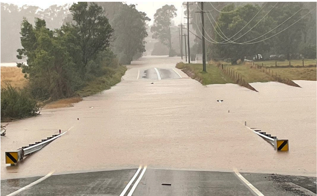
Flood Damage. Source: Wollondilly Shire Council
