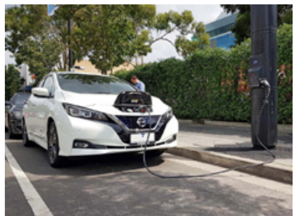
Electric vehicle charging, Western Sydney. Image - (Renew)
